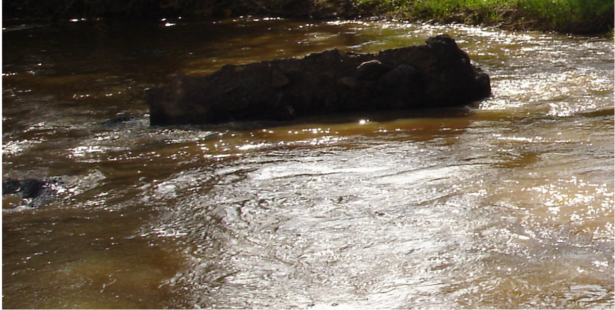
Figure A5: Section of the weir swept away by the floods at 2EG01 gauging station
