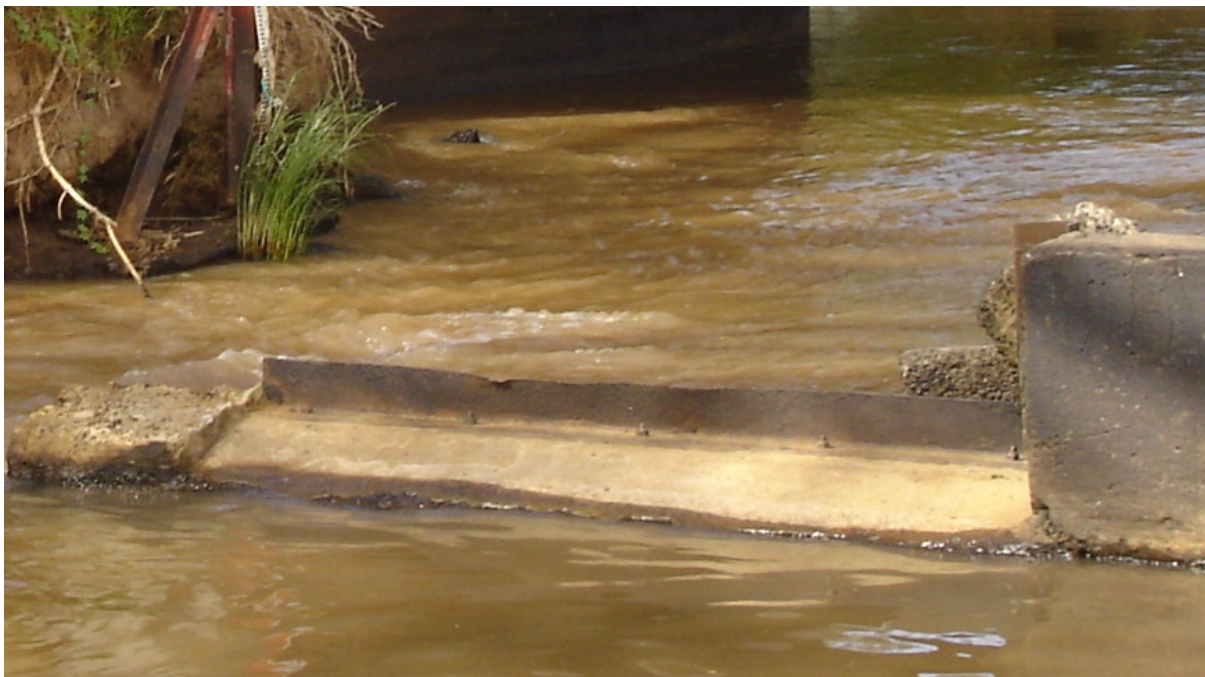
Figure A6: Remaining section of the weir at the catchment outlet 2EG01
