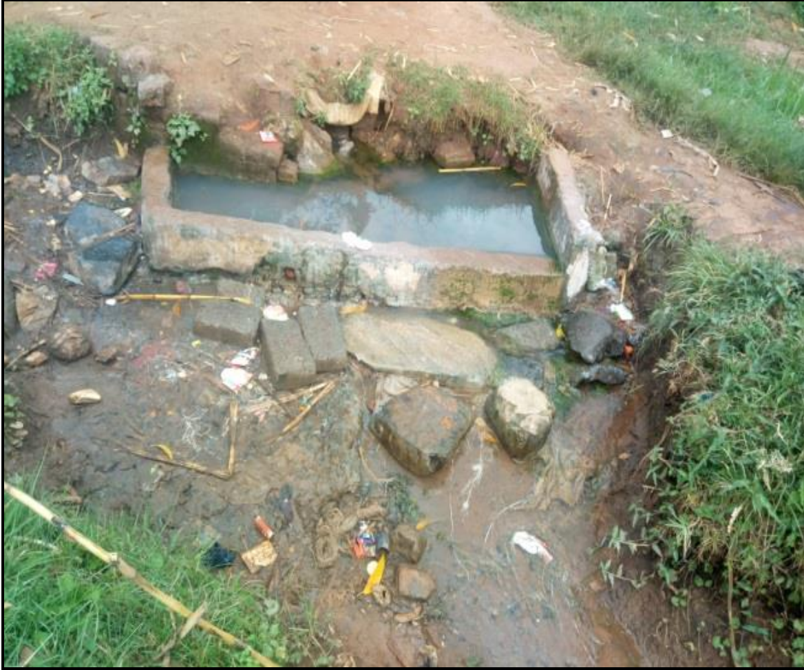
Plate 4.7.3: A Broken and Neglected Natural Spring in Kipsongo Project Site
