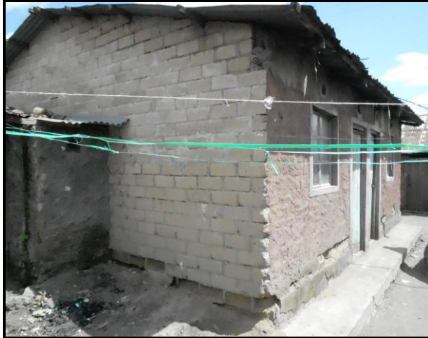
Plate 4.5.8: A Poorly Maintained Low-Cost House in Lake View Project Site
