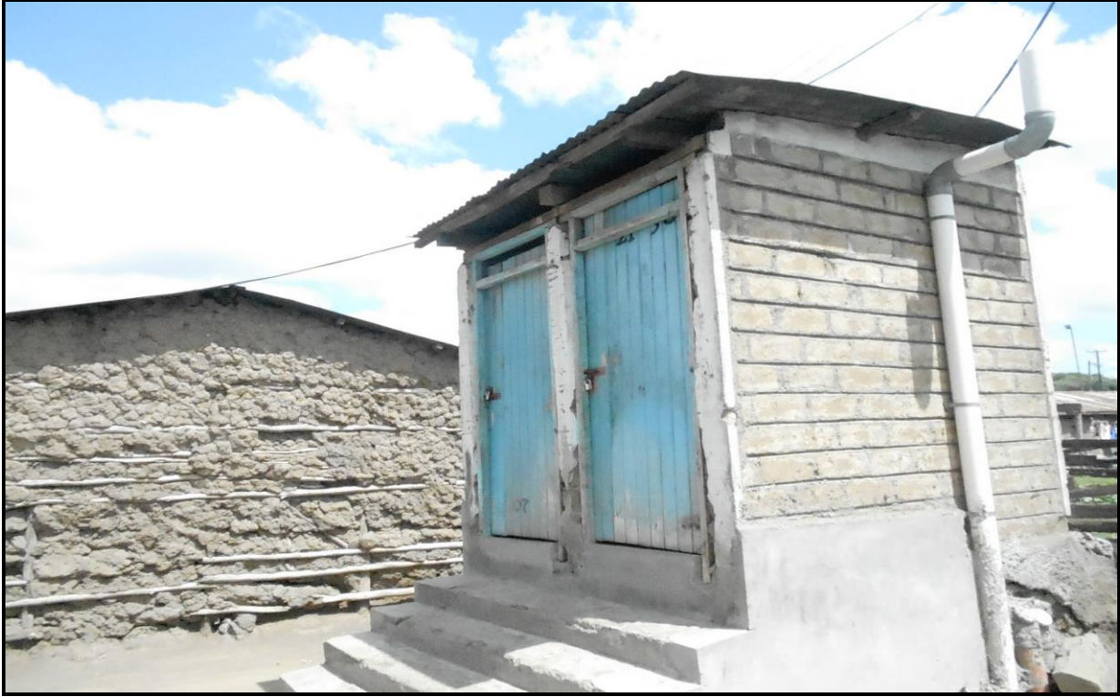
Plate 4.5.16: Abandoned UDDT in Lake View Project Site
