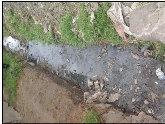
Plate 4.7.7: Blocked Open Sewer in Bondeni Project Site
