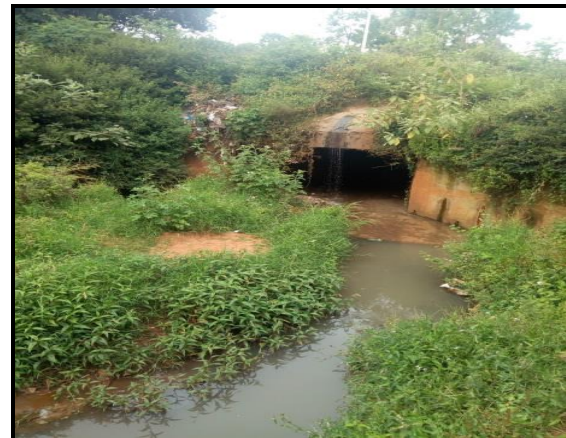
Plate 4.7.8: Dumping of Waste in Tuwan River in Tuwan Project Site
