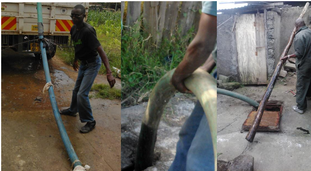
Plate 3: Photos showing desludging practitioners without appropriate PPE
