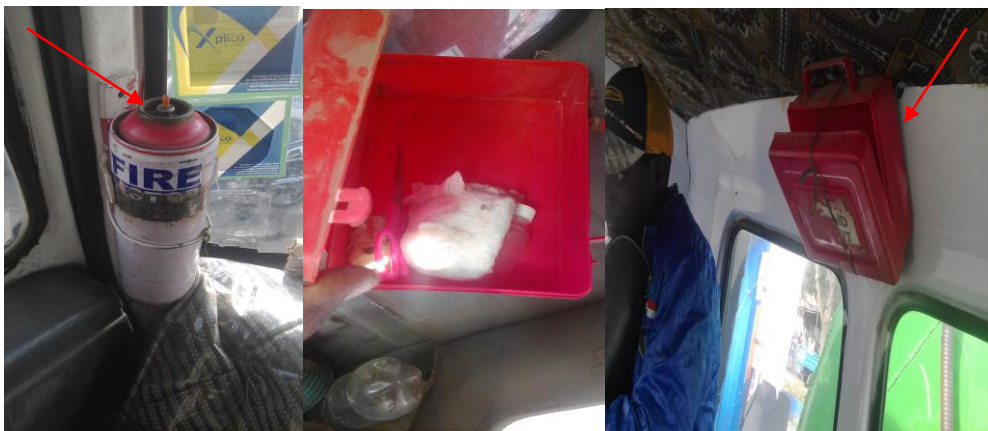
Plate 4: Photos of non functioning fire fighting equipment and empty first aid kits
