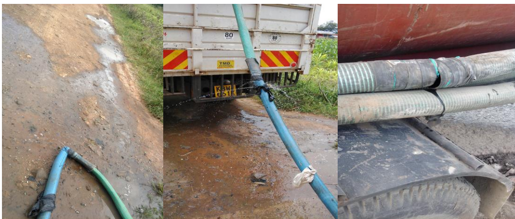
Plate 1: Photos showing worn out and torn suction pipes spilling septage to the environment
