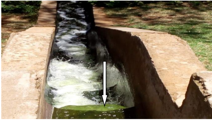
Plate 4.10: Last Maturation Pond of Huruma Sewage Treatment Plant Discharging Poorly Treated Effluent Water into Sosiani River at a Fast Rate.
